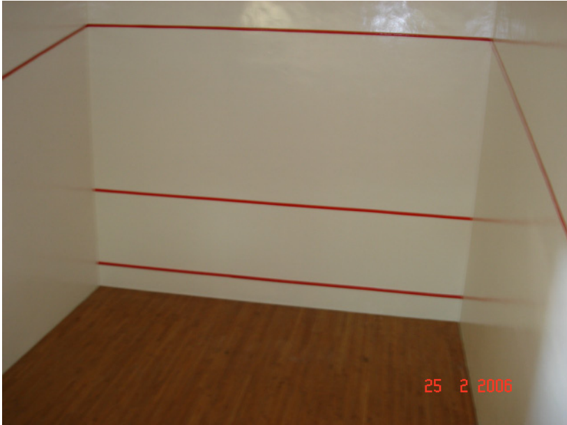
Figure 1. Original state of the two squash courts before the construction and renovation work.
