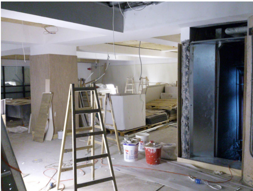
Figure 3. Photo was taken from within the existing weight room. The floor is now complete and the wall that was being removed in Figure 2 is now completely removed. The rough edges of that wall are shown on the right side of the picture, near the air-conditioning duct.
